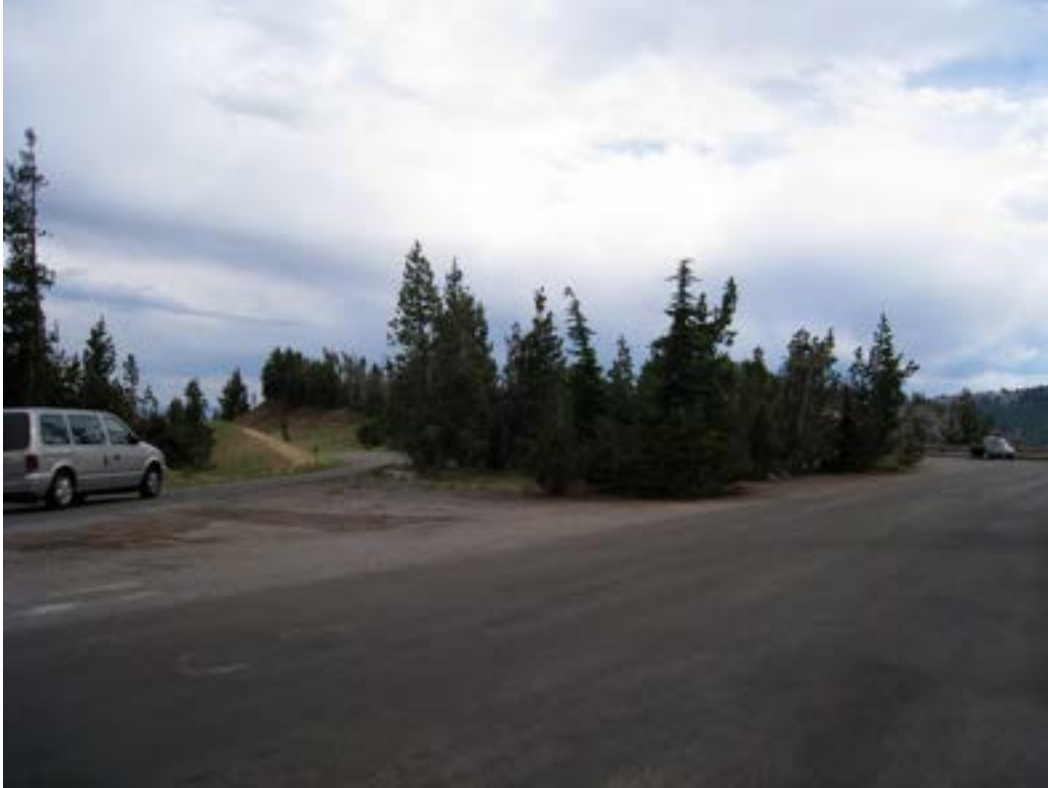
Circulation #15: View of Reflection Point substation (Germano, PWR, 2010).
