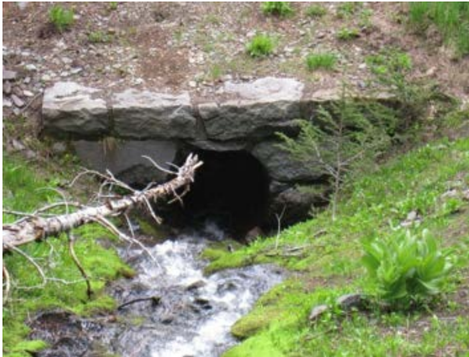
Buildings and Structures #6: Culvert with stone masonry headwall near Sun Creek Valley Vista (Gjesfjeld, PWR, 2010).
