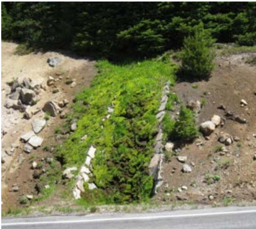
Buildings and Structures #4: Stone masonry spillway overgrown with moss and grass along Rim Drive segment 7-D (Gjesfjeld, PWR, 2010).
