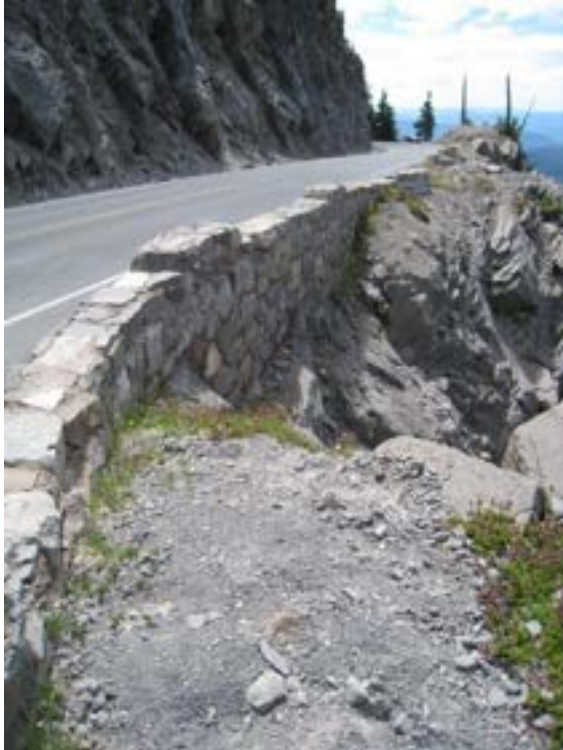
Buildings and Structures #3: Stone masonry retaining wall and guardrail along Rim Drive (Hartzler, PWR, 2008).
