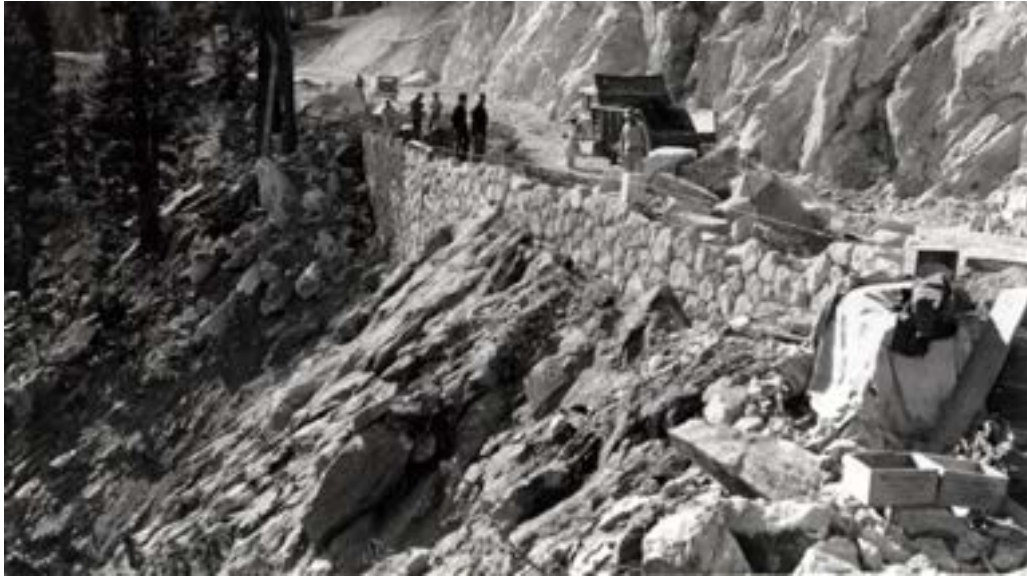
History #3: Construction of a stone masonry retaining wall at Scott Bluffs, 1934 (Doerner, NARA, RG 79, SB).
