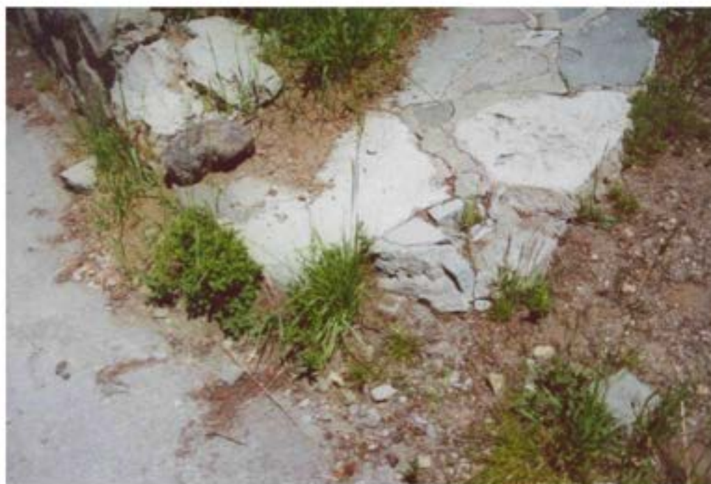
Contemporary photograph showing the condition of the flagstone walkway at the front of the residence. Impacts from severe weather conditions have eroded the mortar bonds, causing joints to fail. (CCSO, 2000.)
