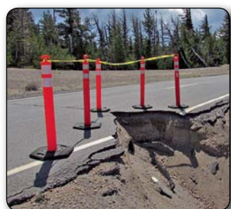
Built in the 1930s, Rim Drive is long overdue for repair. In 2014, part of the East Rim Drive began eroding into the caldera.
