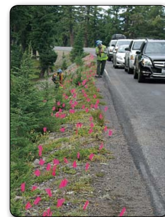
The world’s largest known population of Crater Lake rockcress grows along the West Rim Drive. Road construction will displace it temporarily. In 2014, prior to rescuing some of the plants, employees conducted a census by marking each one with a pink flag. They counted 1,927!
